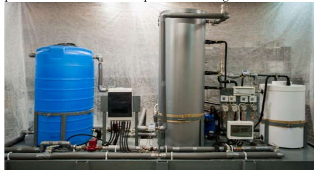
Figure 1. Appearance of a multifunctional thermal point at the test bench
